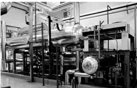
Beauvais CO 2 / NH 3 machine room.
